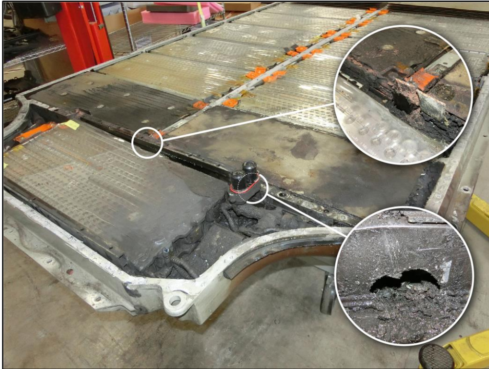
Figure 15. Battery pack with top cover removed to show location of holes in battery case and insets showing closeups of damaged areas.
